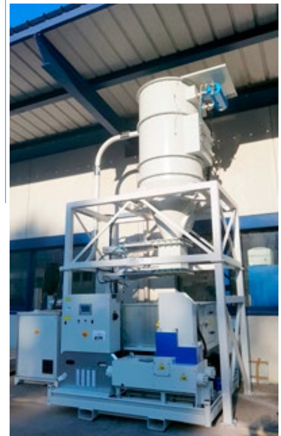
Vacuum plant feeding a briquetting machine
