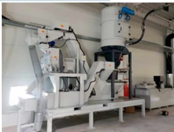
Vacuum plant discharging into a spinning system
