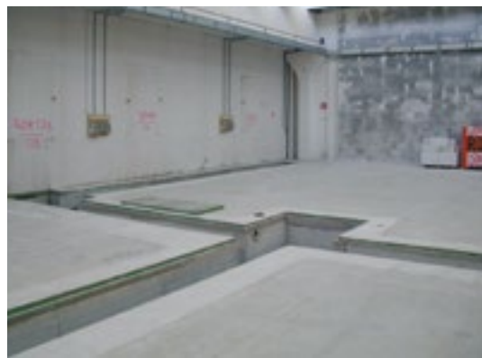
Detail of in-ground lines
