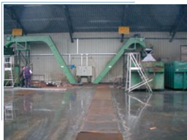
Aluminium conveying line
